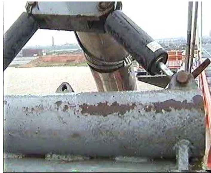
Details of Magnetorheological fluid damper in Dongtinghu Bridge
