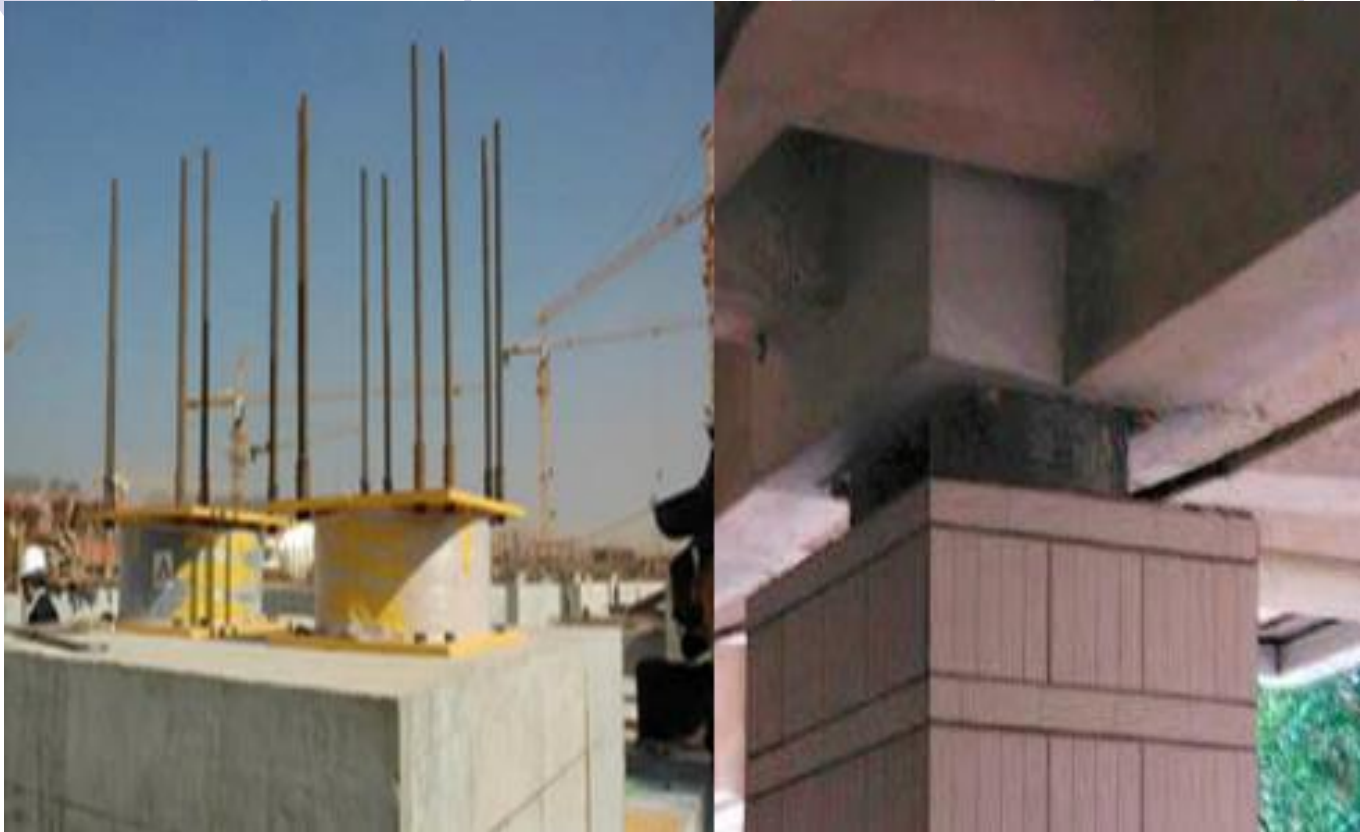
Isolators in bridge
